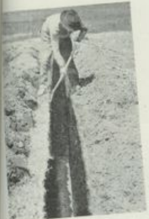
Soil covering the tile with slack dirt as soon as they are laid.
