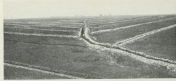
A tile system with the main ditch dug up a central drain, the laterals coming into it from both sides on the "Herring Bone" plan.
