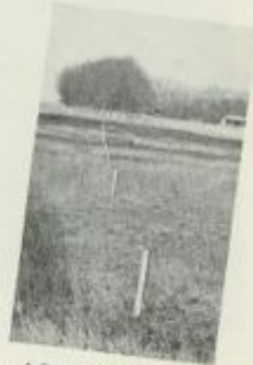
A line of stakes set by the engineers for the guidance of the diggers.
